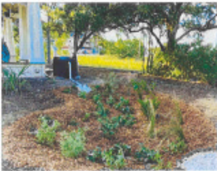
Rain Gardens with Cistern
