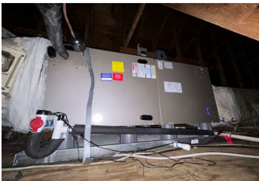
2 nd Floor East Side AHU in Attic
