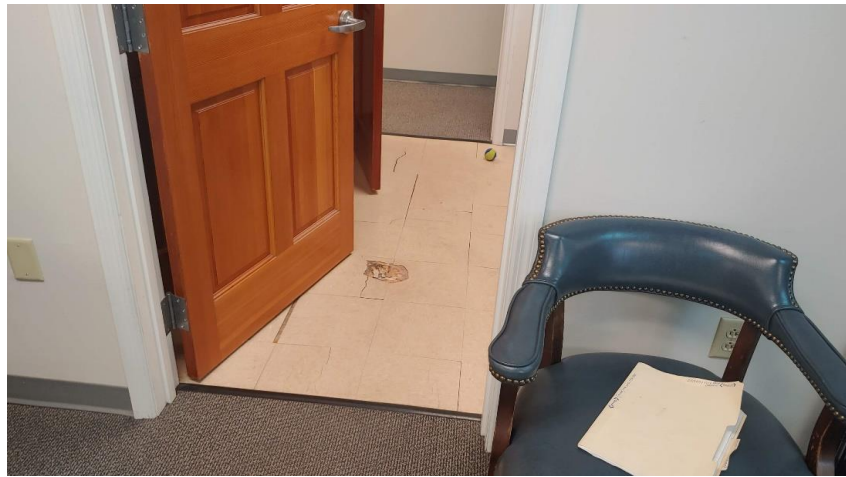
Photograph No. 5 Water damage to floor: below HVAC Unit
