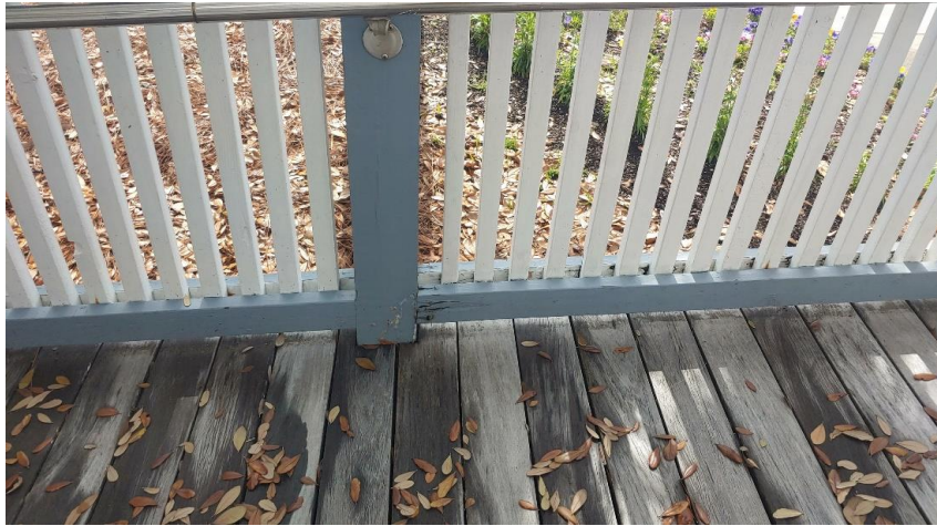
Photograph No. 17 Guardrail at First Floor Level, Note deterioration.
