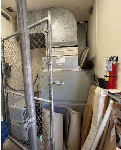
1 st Floor West AHU in Mech/Elev Rm
