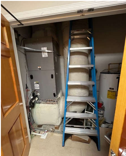
1 st Floor East Side Mech Room
