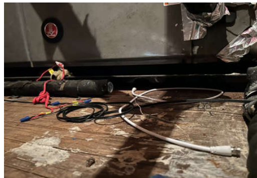
2 nd Floor West Side AHU in Attic
