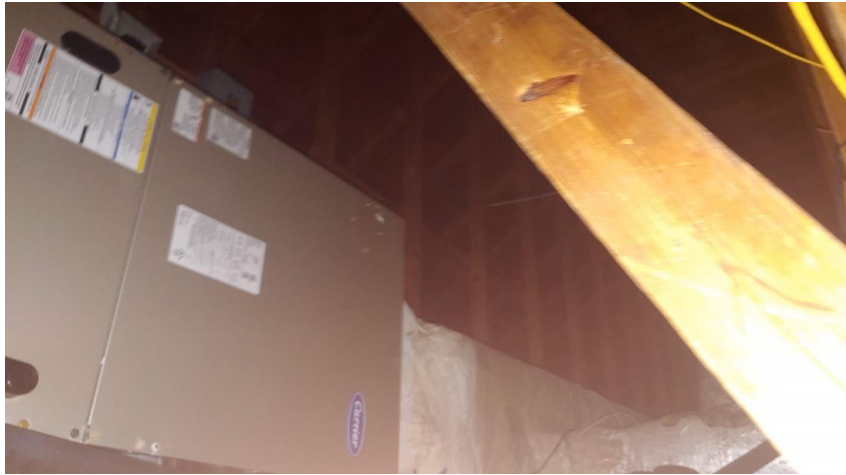
Photograph No. 3 HVAC Unit above ceiling, supported by Roof Trusses
