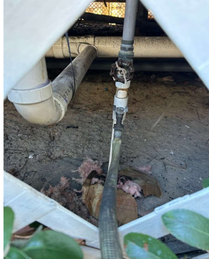
2 nd Floor Sink @ Conf Room
