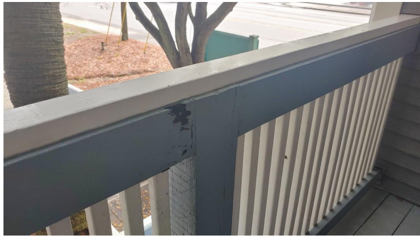
Photograph No. 15 Guardrail at Second Floor Level, Note deterioration.
