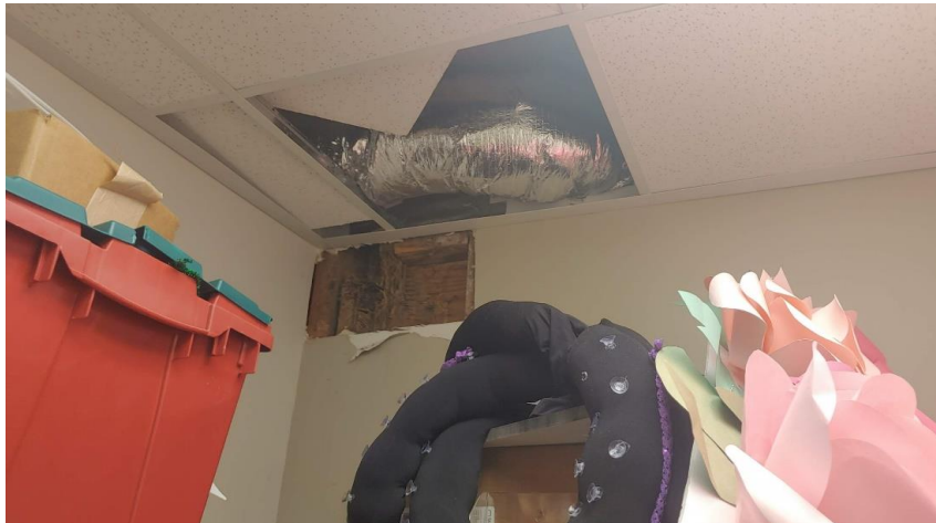
Photograph No. 4 Deteriorated Wall Framing below HVAC Unit
