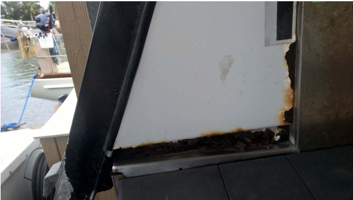
Corroded Fuel Dispenser - Beyond Repair
