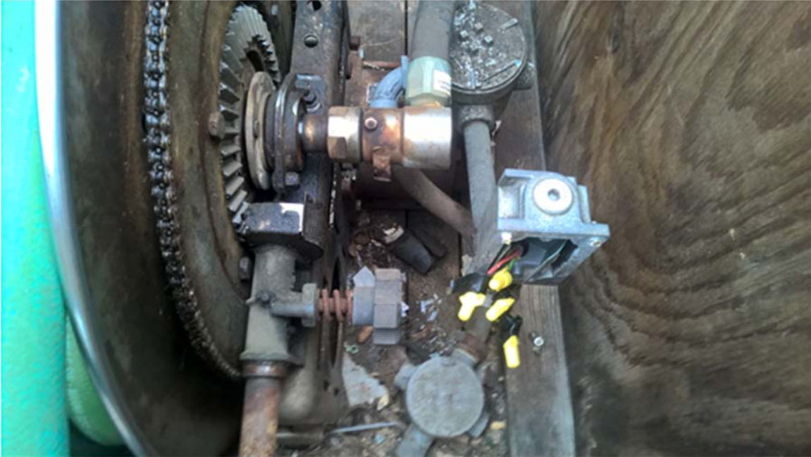
Improperly Sealed Junction Box in Marine Hose Reel = Explosion Danger
