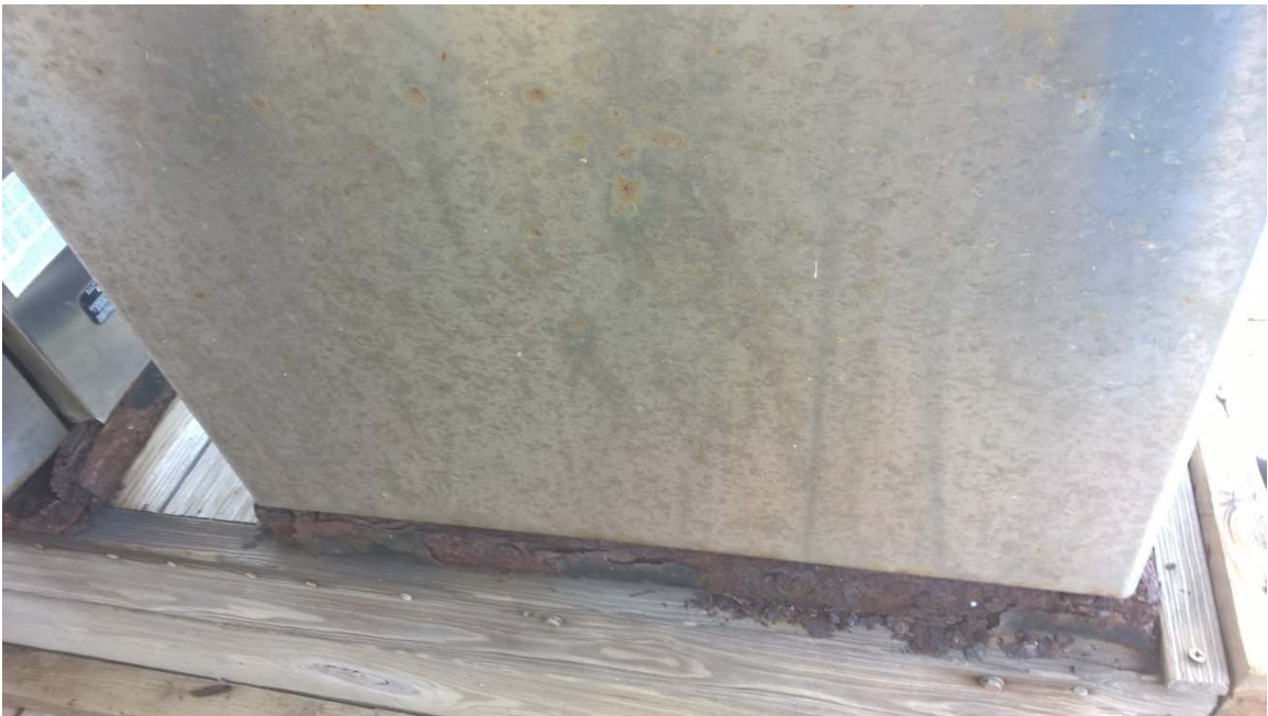
Corroded Fuel Dispenser Base - Beyond Repair
