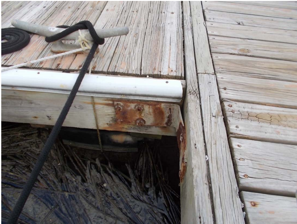
Failing Dock Connection Hardware
