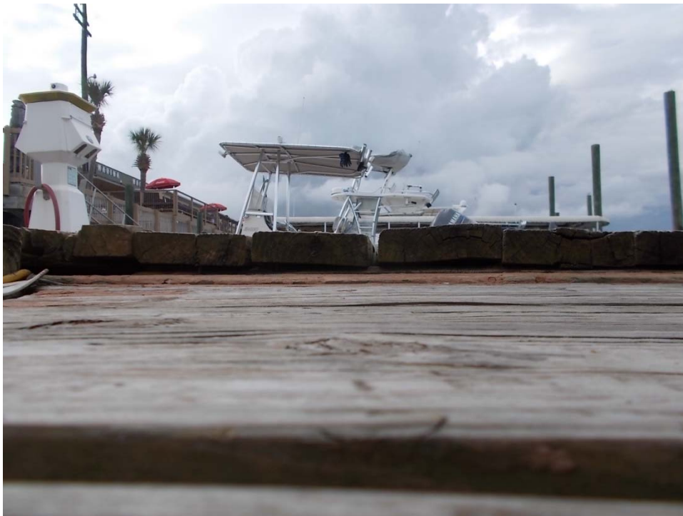
Uneven Deck/Framing Failure at Existing Fuel Dock
