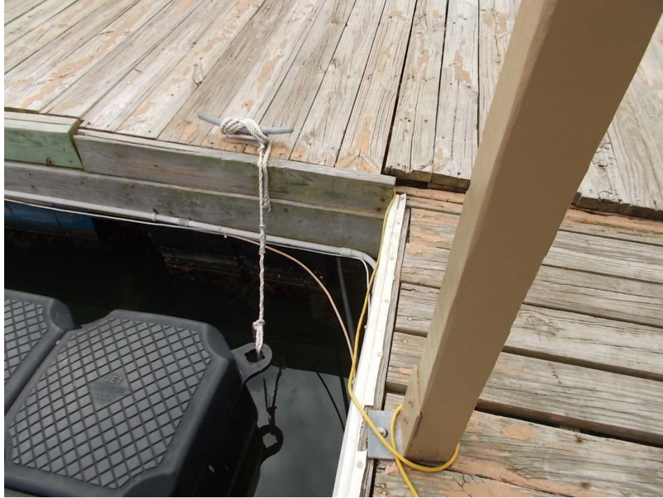
Framing Deterioration, Lack of Sub-Deck Conduit Space, Limited Fuel Hut Anchorage to Dock
