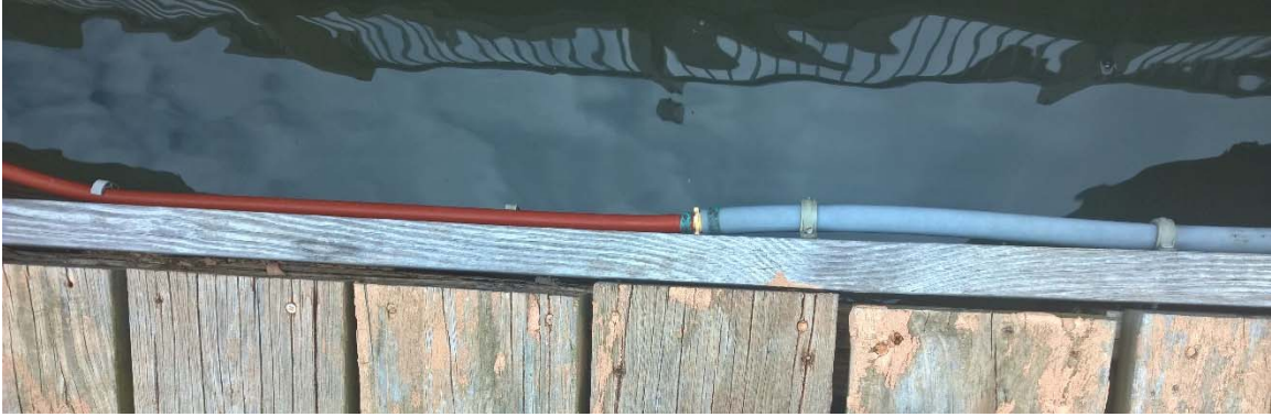
Different Types of Piping and Different Sizes Connected (Lack of In-Dock Conduit Space)
