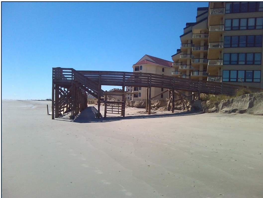
FIGURE 3.38. The boardwalk at the Ocean Club complex following passage of Hurricane Sandy in October 2012. Since this photo was taken, a small volume of sand from upland sources has been placed by property owners to rebuild the dune.
