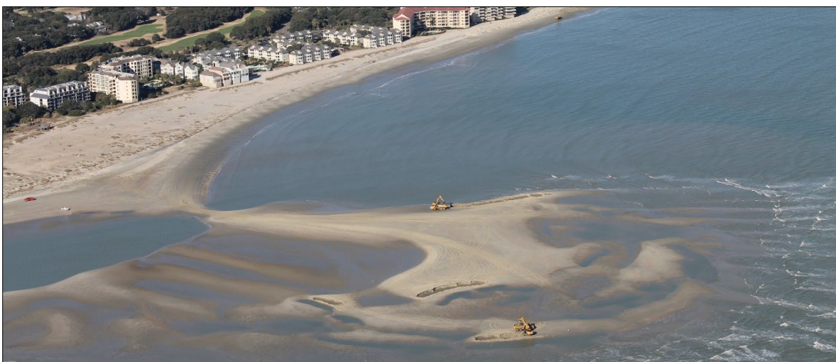
FIGURE 2.10. January 2015 aerial image of the 2014–2015 shoal management project showing equipment transferring sand from an attaching shoal to the eroded beach.
